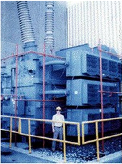
PJM Public Service Step Up Transformer
